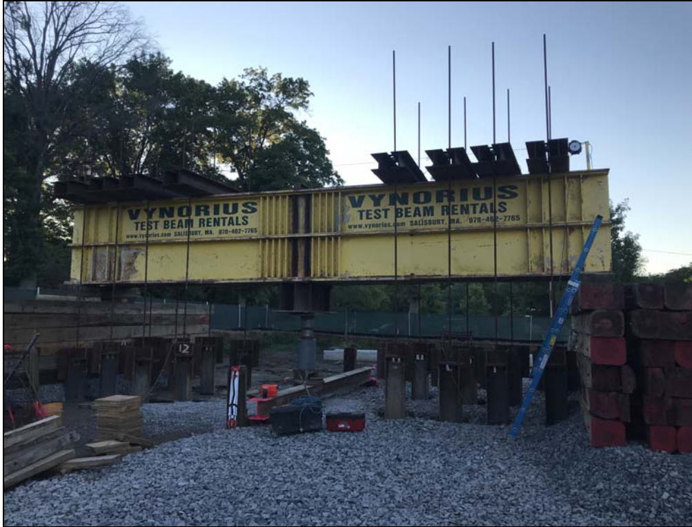
Figure 3 – Large Static Load Test Frame For 500 ton Compression Test Load (photo courtesy of GTR)
