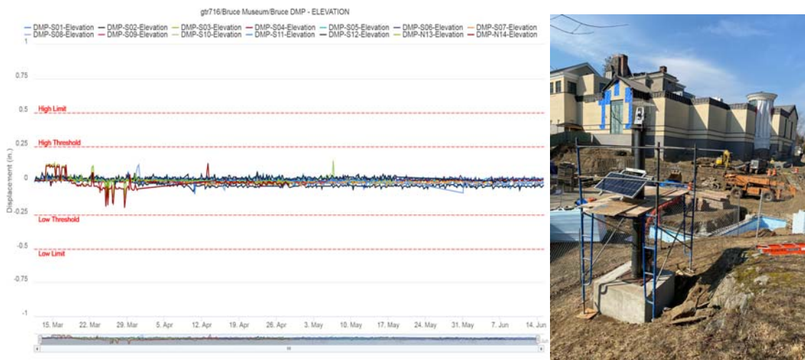
Figure 5: Elevation data of existing structure behind soil nail wall through the monitoring program and one of the AMTS setups at the project.
